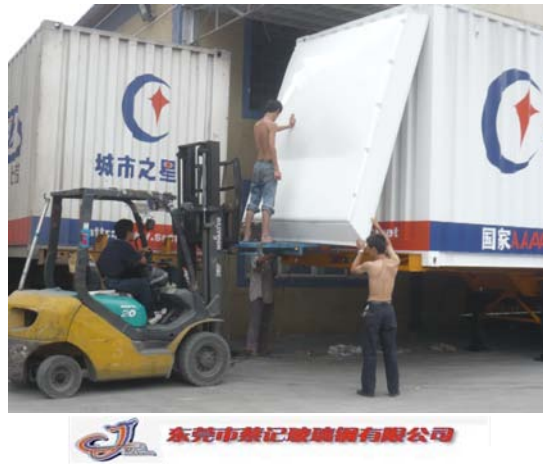
Figure 4: Nose cones of the brand DongGuan CAIJ installed on HDTs
